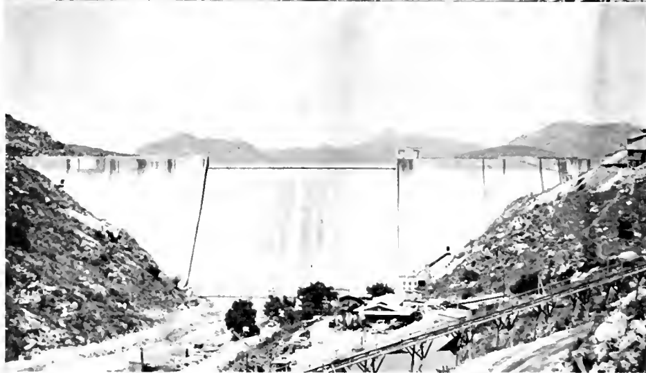
San Vicente dam under construction across highway showing hole left for traffic during road relocation. At bottom, the completed dam
